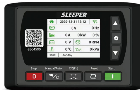
Generator Control Panel
